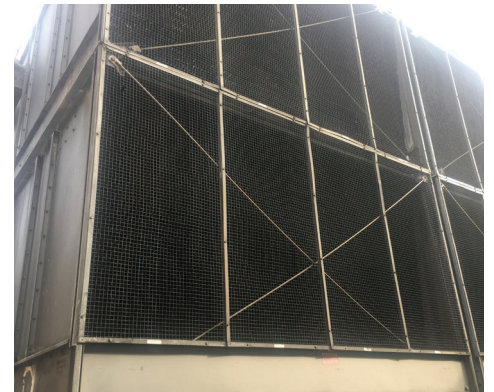
Condenser system at Perkins Rowe site.
